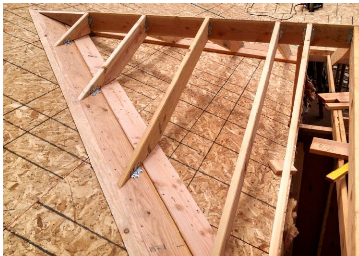
Valleyboard/Ledger board to be one size larger and must support the rafters (see example above)
